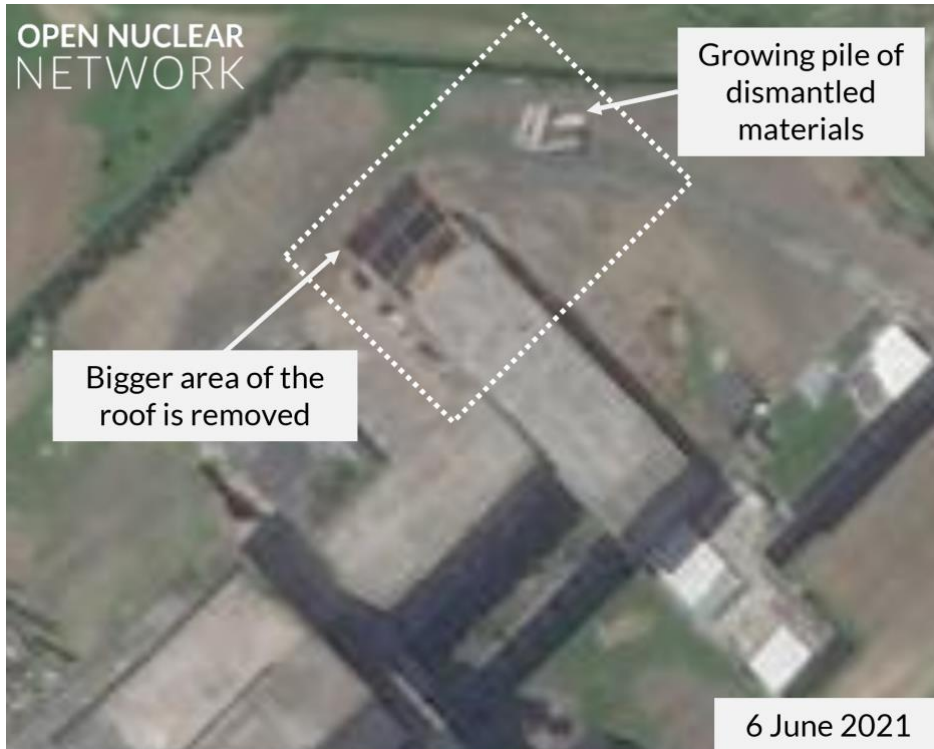
Figure 2. Further dismantlement of the roof detected in satellite imagery from 6 June 2021. Image © 2021 Planet Labs Inc. All Rights Reserved. Reprinted by permission.
